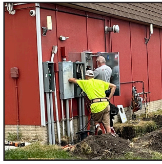
G&R Electric installed a new 600-amp electrical service to the Main Barn.
