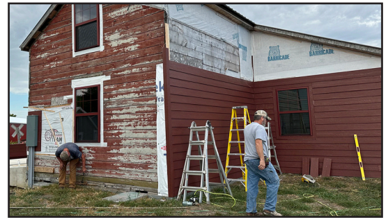
Aaron & Sons was the general contractor for the installation of siding on the railroad Section Foreman's House. Wheels volunteers assisted.
