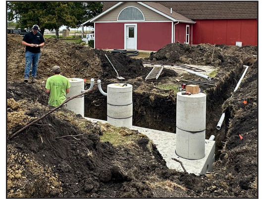
A large capacity septic tank was put in place this summer by ET Heating & Cooling.
